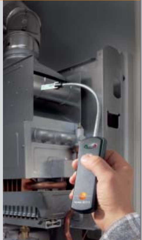
Establishes if flue gases have been drawn off completely from the burner
