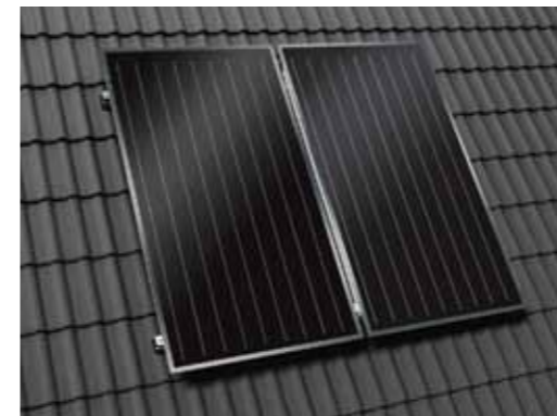
Solar-Lito on-roof installation
