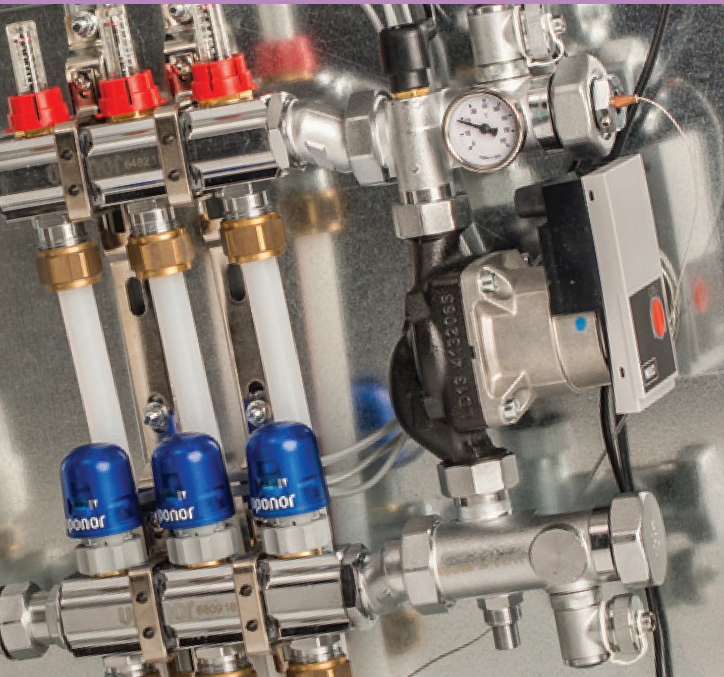
Water Temperature Control
