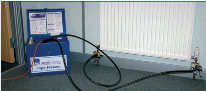
Fig. 1. Shows Arctic Electric ready to isolate the radiator in order to change the radiator valves.
